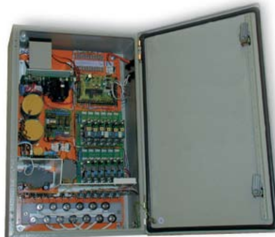
Z6 Control Cabinet
